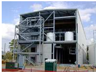
Figure 2.9. Main Process Building of TVA Flow Battery [43]
