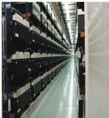
Figure 2.7. NiCad Battery Energy Storage in Fairbanks, Alaska [18]
